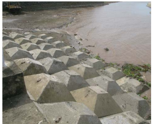
Shoreline protection in Vietnam.
