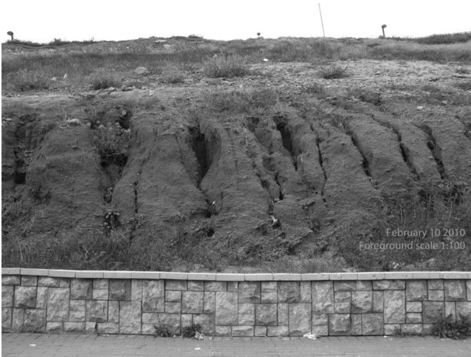
Figure 3. Close-up eastward view of cliff erosion affected by surface runoff held back by retaining wall within Segment K (high erosion). Cliff height: \sim 20 m.
